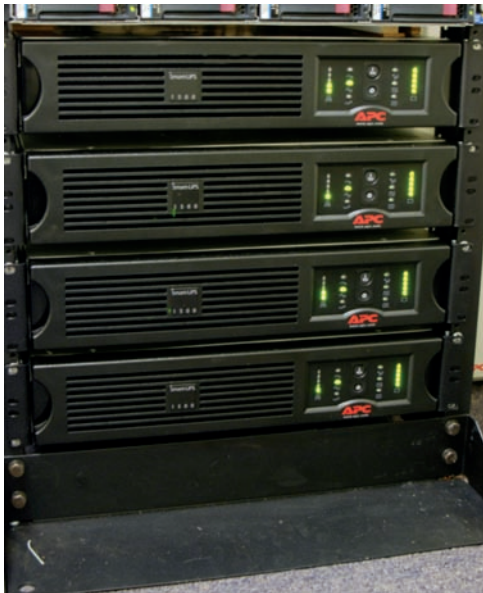
Figure 11-30 Online UPSes installed on a rack
