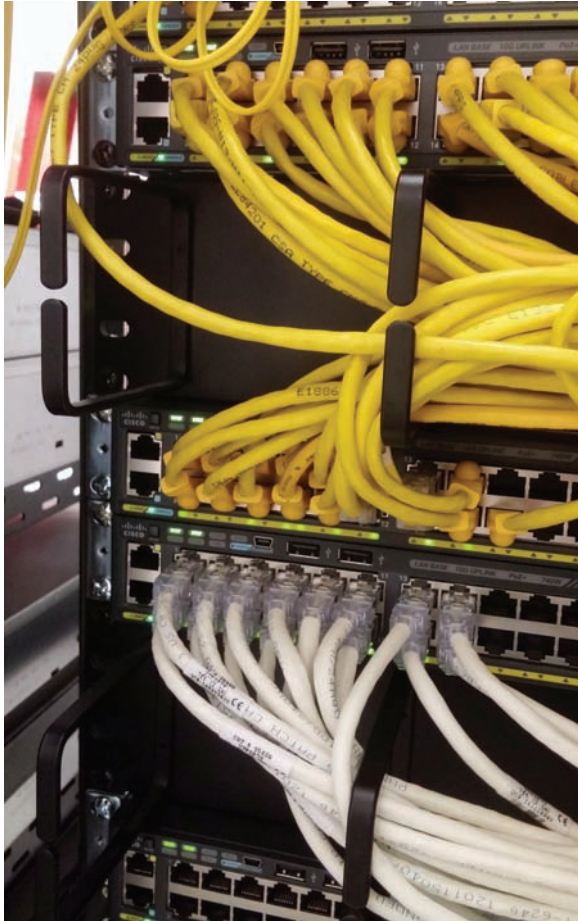
Figure 2-19 Cable management brackets installed on a rack
