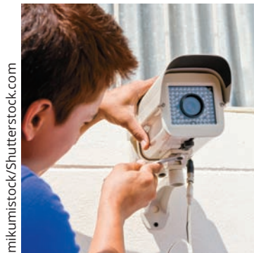
Figure 9-18 IT personnel might be responsible for the installation and maintenance of a CCTV network
