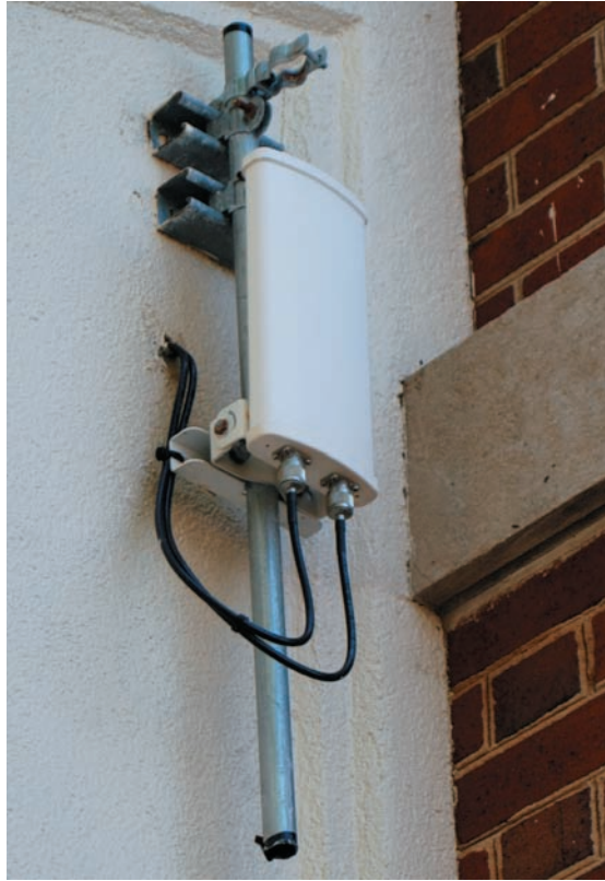
Figure 6-27 An outdoor unidirectional antenna that transmits across a nearby football field
