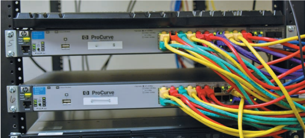
Figure 2-20 Different colors of cables can indicate the general purpose of each cable
