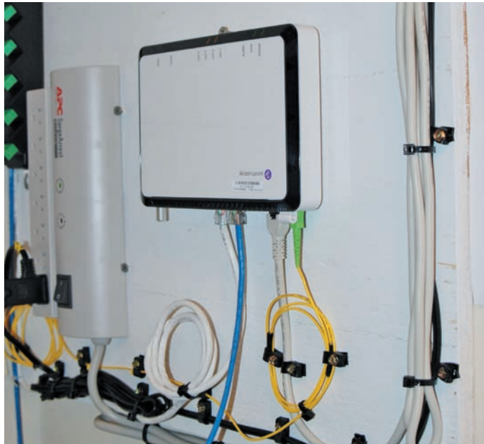
Figure 2-3 Demarc for Internet service to a campus network; this demarc is located inside a small data room and is mounted to a wall near two racks that house routers, switches, servers, and UPSes
