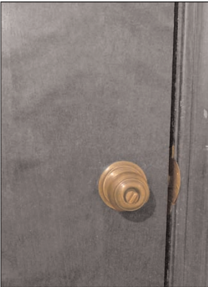
FIGURE 7.6 The lock adds minimal security, and the door can still be opened rather easily.
