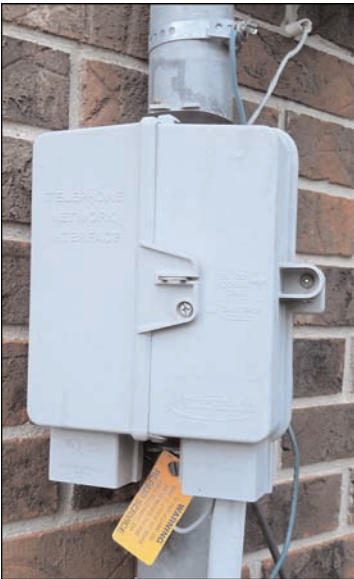
FIGURE 5.5 The point of demarc for a home.
