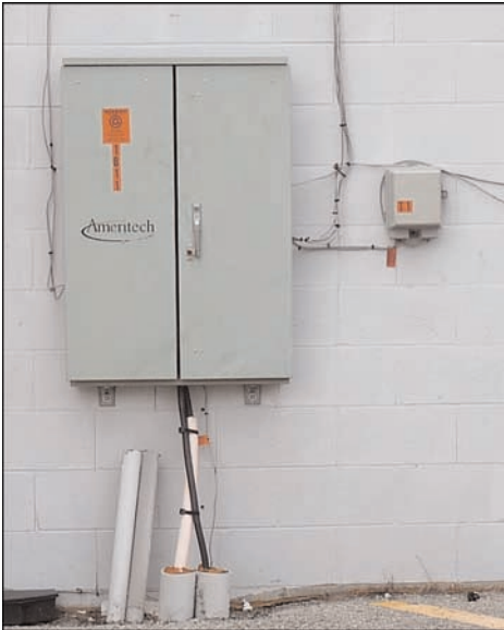
FIGURE 5.6 The point of demarc for a small office.
